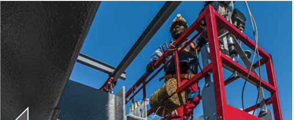
4m Temporary Suspended Platform on the ABSA Towers Redevelopment Project, Johannesburg CBD.
